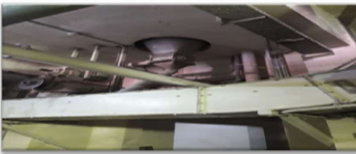
Figure (1) Distribution Assembly and Motorized Valve System
